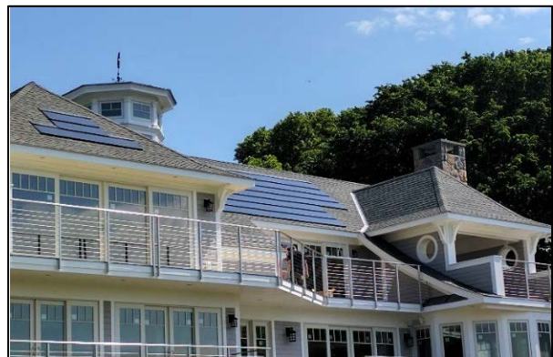
The awarded SunTegra solar shingle roof installed with Murphy Brothers Contracting in Stamford
